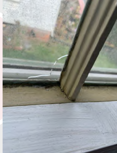
Front bed side window cracked glass
