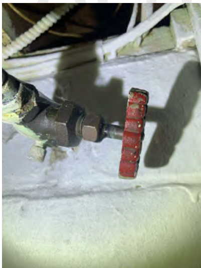
Leaking valve above washing machine
