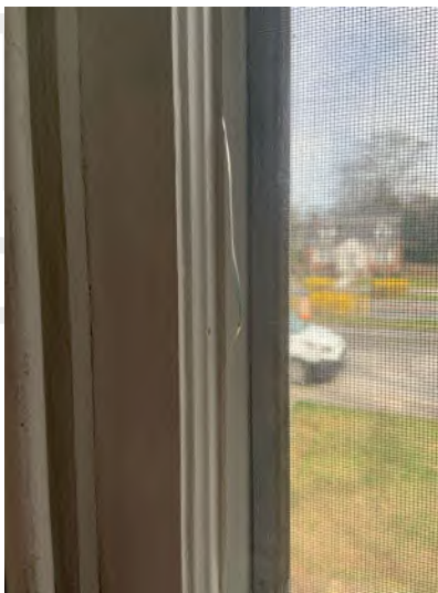
Front window cracked glass
