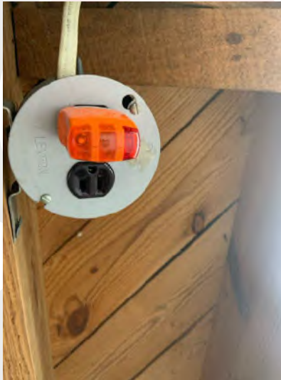
Ceiling outlet not enough power
