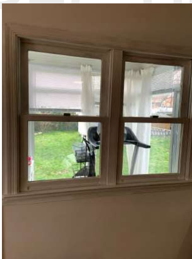
Left window top pane paint shut / right window top and bottom panes slide down
