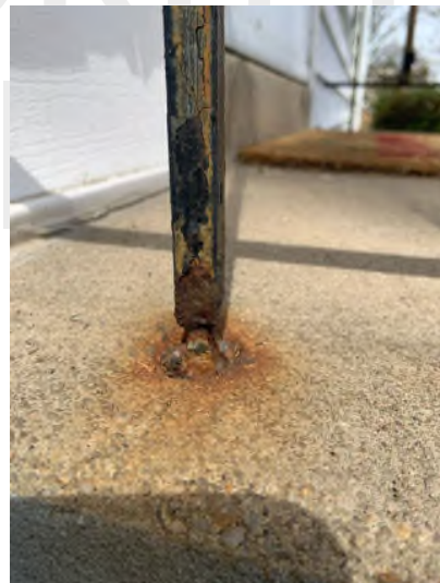
Guardrail pole rusting out
