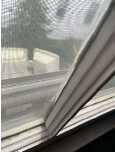
Glazing coming off when opening and closing
