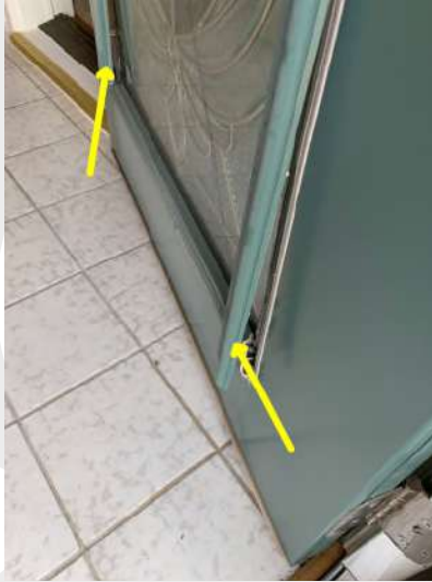
Front door trim is coming off
