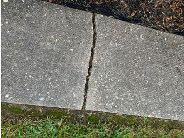
Crack noted in sidewalk
