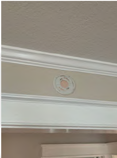
Missing smoke detector noted
