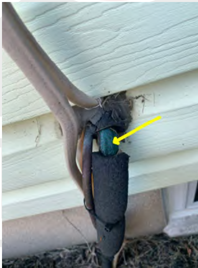
Missing insulation noted
