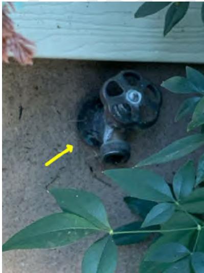
Recommend sealing around front hose bib
