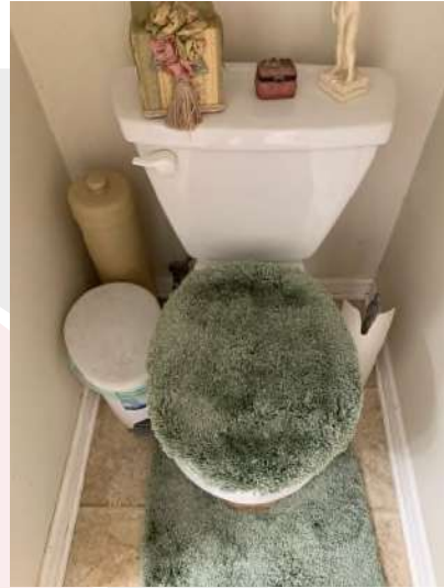
Basement toilet is loose to the floor
