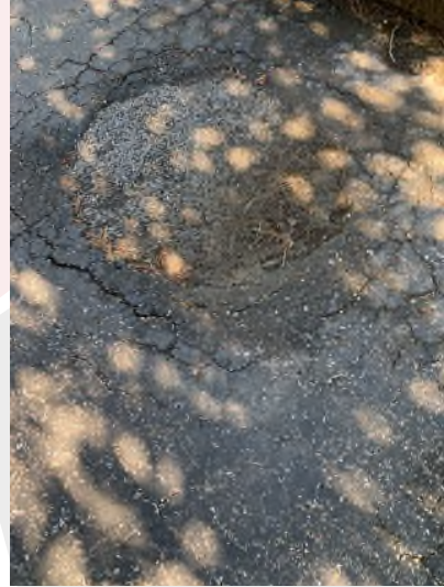
Cracks and damage noted in driveway
