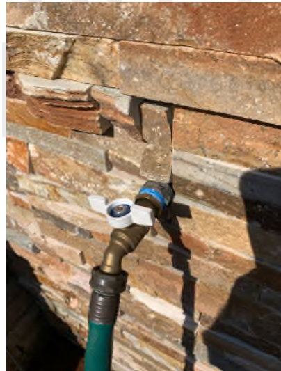
Rear faucet is loose
