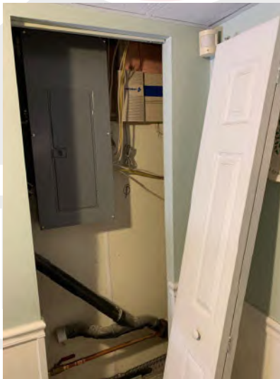
Closet door is off the tracks
