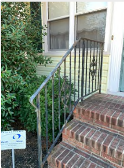
Loose handrail noted at front steps
