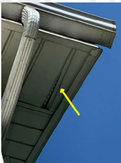
Loose soffit noted at rear of house
