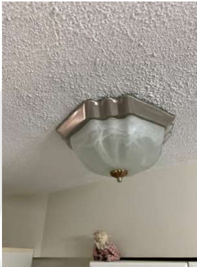
Light is inoperable
