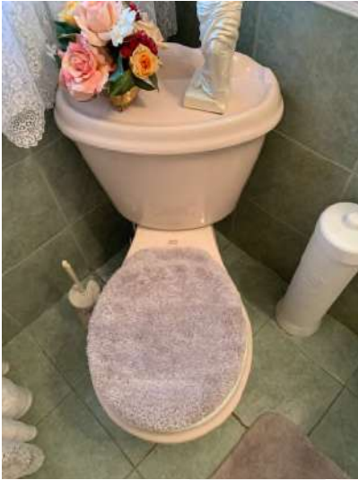
Upstairs bathroom toilet does not flush
