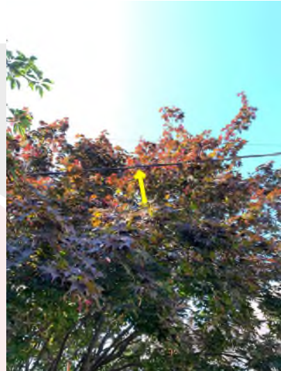
Service cable is touching trees
