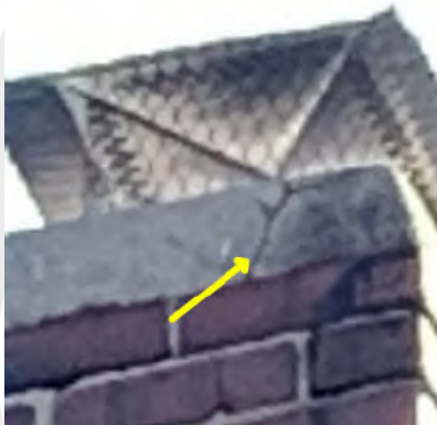
Crack noted in crown
