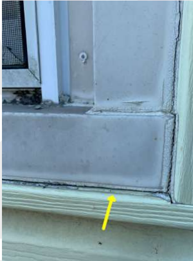
Cracked caulk noted
